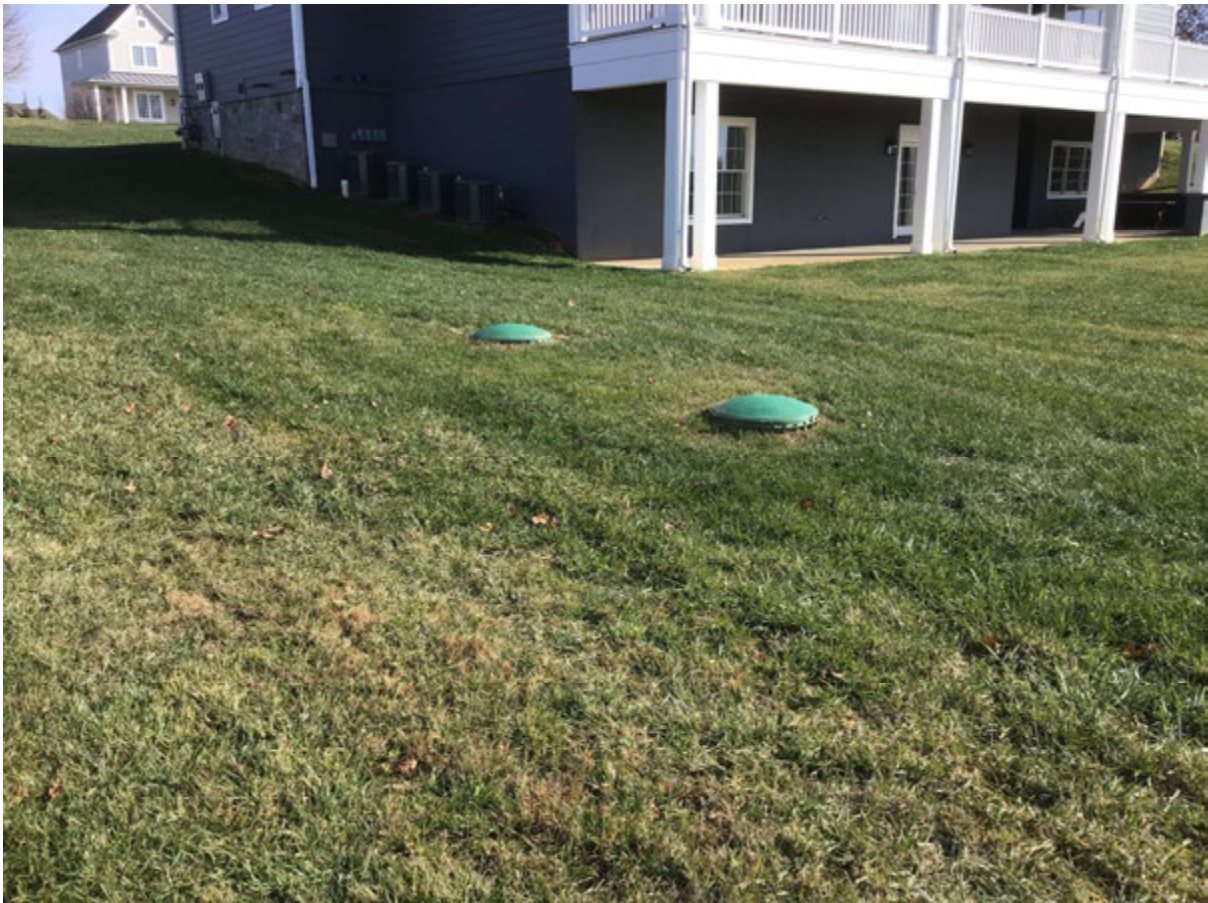
A recently installed, properly graded septic tank with manhole risers to grade.
