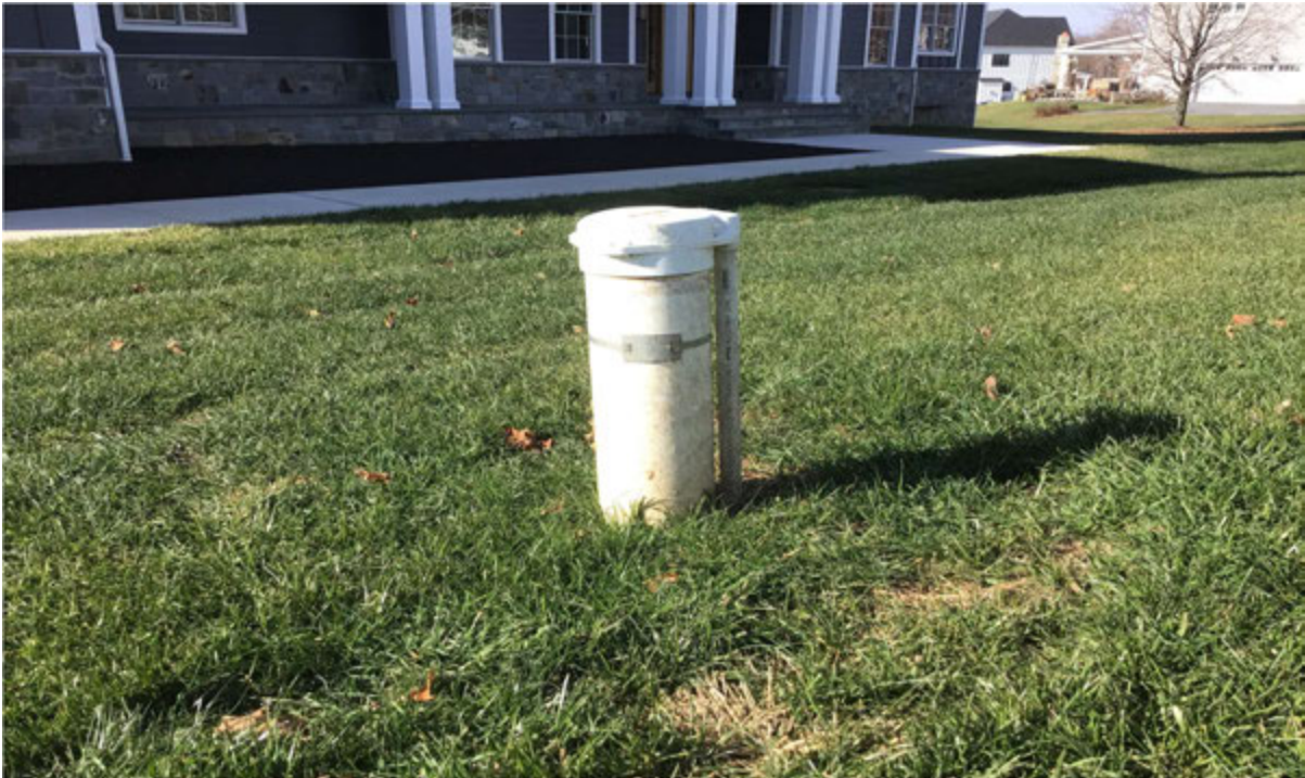
Well casing with a properly sealed sanitary cap, electrical conduit, and state identification tag securely affixed.
