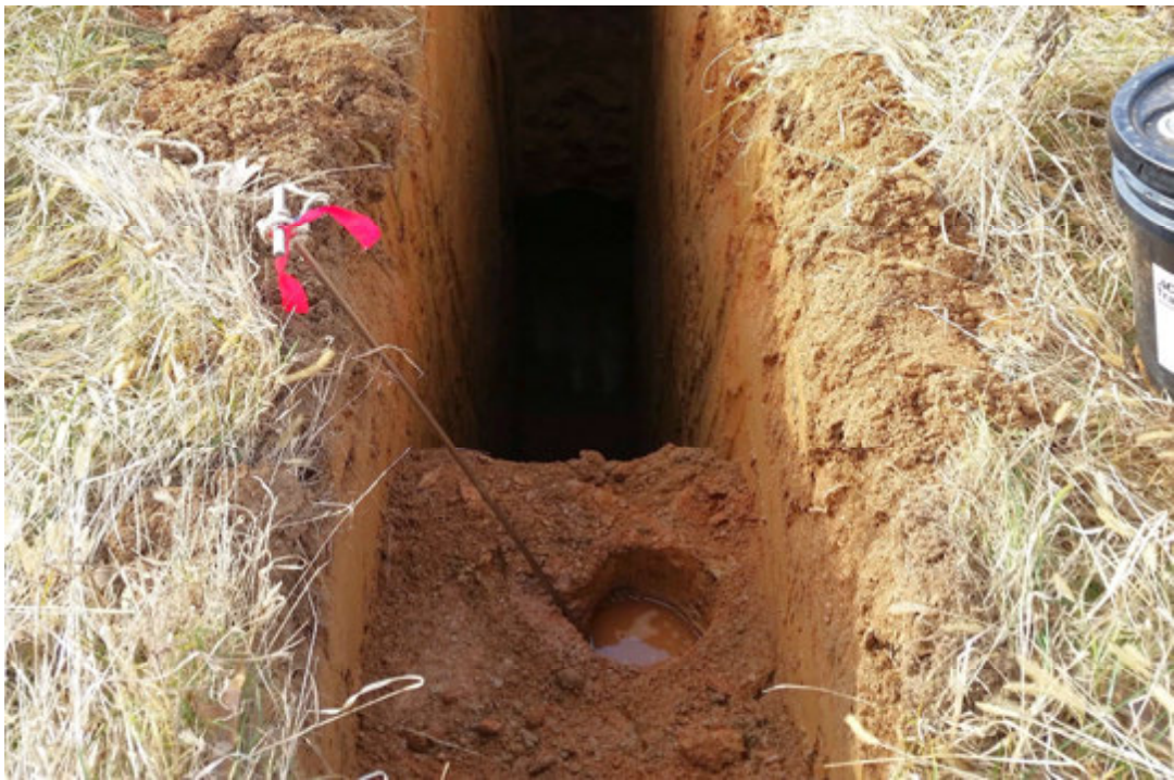
Example of a standard water test being performed to determine the soil permeability rate.
